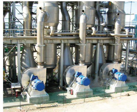
MVR blowers for zero liquid discharge
