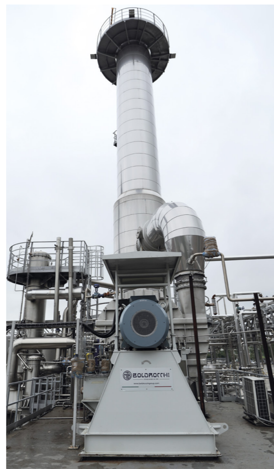
MVR blower for tomato processing plant
